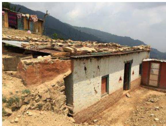
Figure 3.23. One of the houses in Chalal Ganeshthan Ward 9 where the upper floors were demolished and the ground floor level covered with CGI sheets.
