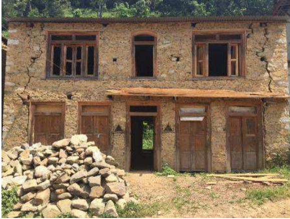
Figure 3.19. Corner cracks of Sita Ram House (builder).
