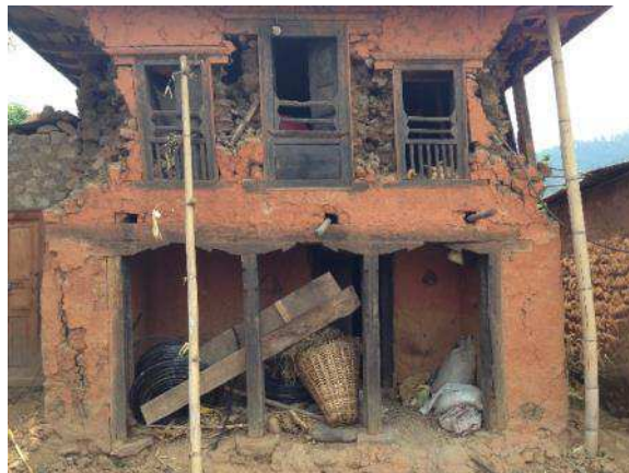
Figure 3.21. Damaged two story house in Mahankal Chaur
