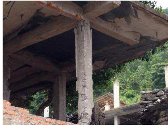
Figure 4.2. Damaged framed infill house, Maneshwor
