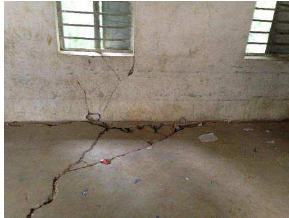
Figure 3.22. School building with cracks in Chyasingkharka.
