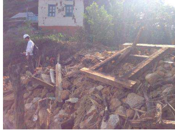
Figure 3.20. Complete collapse of Keshab Prasad's house
