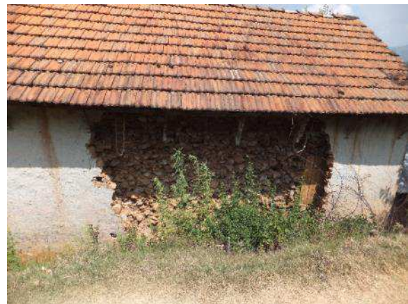
Figure 3.18. Out of plane wall failure of Cheta Nath's house
