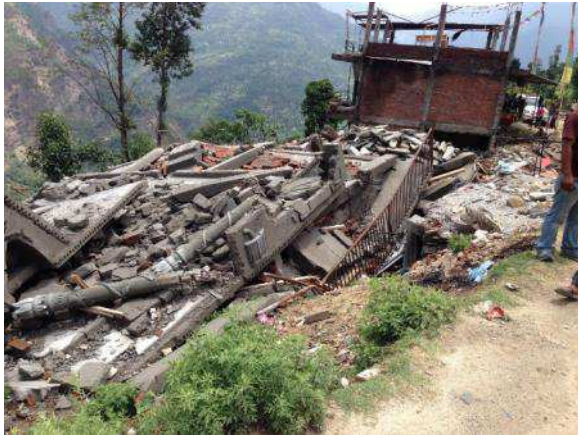
Figure 4.1. Collapsed framed infill house, Maneshwor
